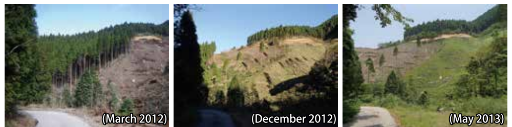
Slope in the process of cutting and forestation (No.102-10 and No.102-13 forest)
